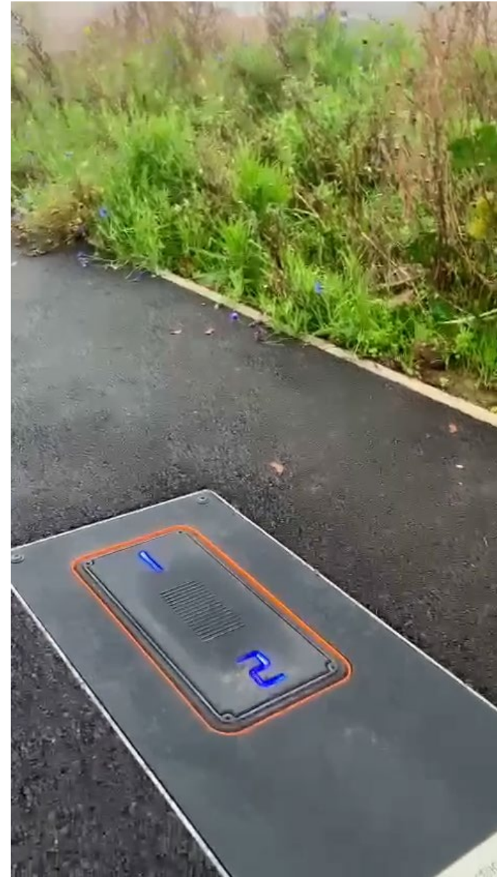
Staffordshire County Council Live Labs EV charger Trial located in Holmcroft Library Stafford (7kWh)
